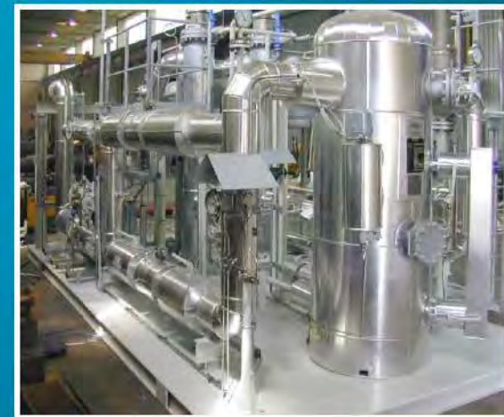
FUEL GAS PACKAGE FOR GAS INJECTION STATION # 300
