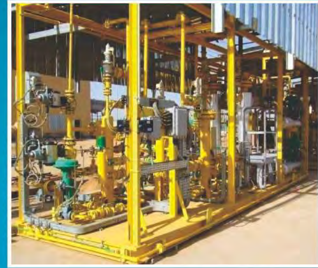
PRESSURE REDUCING 62+20bar. FLOW 2.250 NM 3 /h, 3" PIPING
