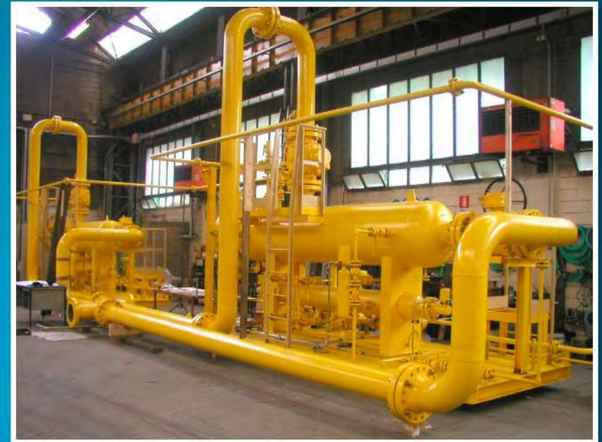
FUEL GAS TREATMENT SYSTEM FOR 750MW COMBINED CYCLE POWER PLANT
