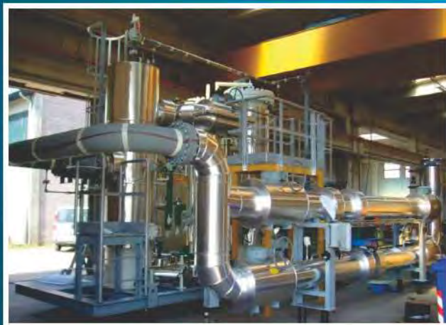
VOLUMETRIC METERING DN 10" # 300 RF
