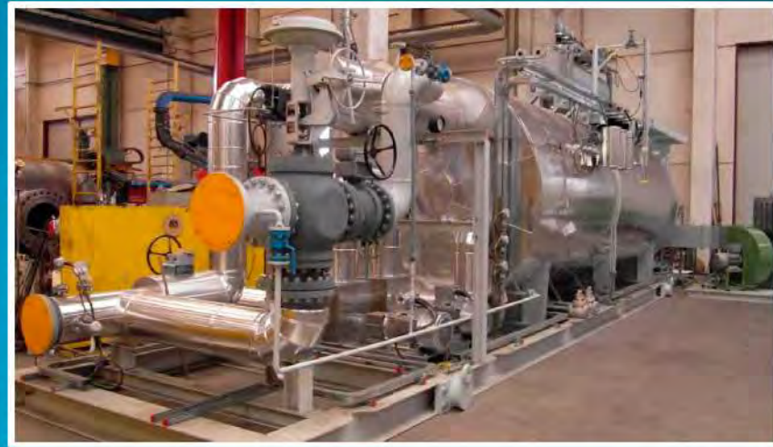
4 FORCED DRAFT OIL BATH HEATERS – 5.500.000 KCAL/h each OIL BATH TEMP. 220° C – OUTPUT GAS TEMP. 126.7° C
