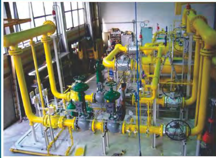
PRESSURE REDUCING 48+36 bar. FLOW 70.000 NM 3 /h, 14" PIPING
