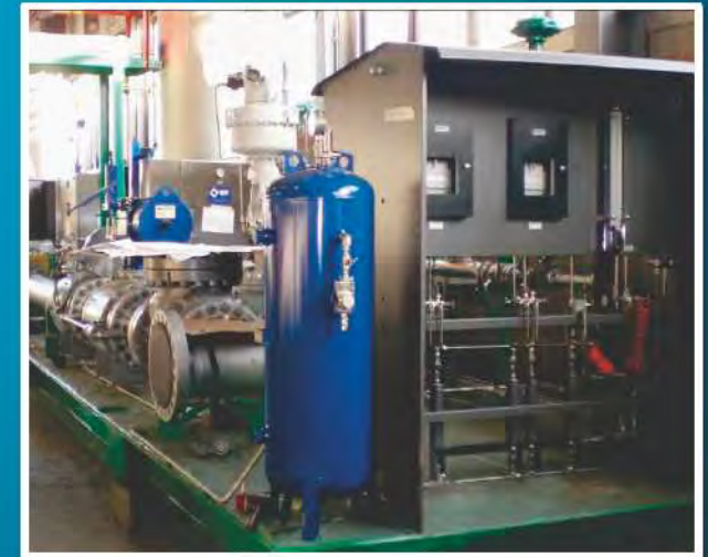
FISCAL METERING DN 14" # 600 RJ
